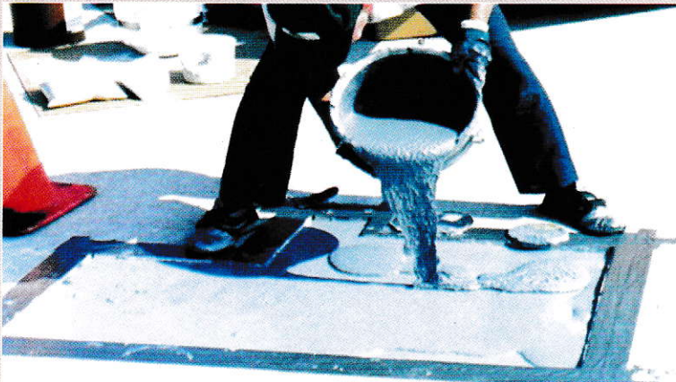
Application: Pouring of Mixed Material on the Surface and Finishing with Trowel for Smoothing & Finishing
